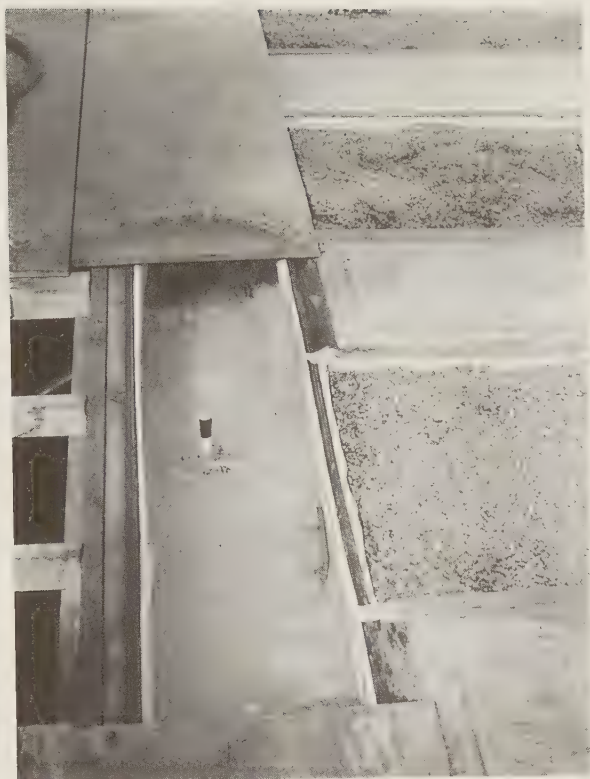
FIGURE 7.6 Bed fill-drain pipe entering plenum.
